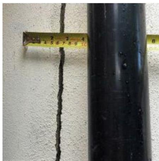
Crack on rear wall.
