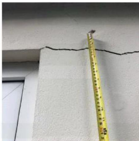
Crack above rear door.
